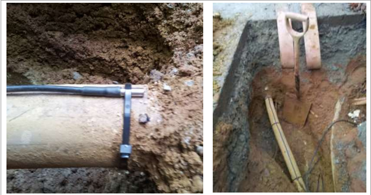
Figure 11: 11kV cable temperature measurement sensor
