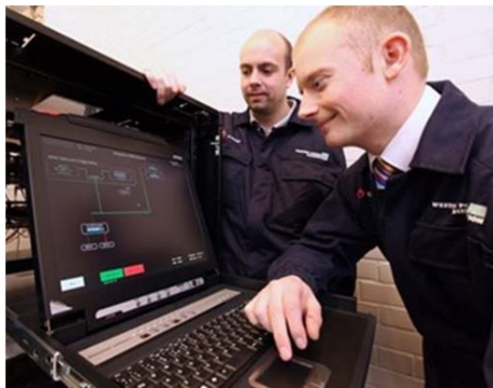
Figure 4 – Active Network Management installed at Skegness Grid Substation
