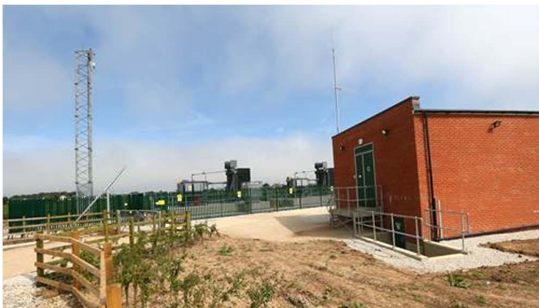
Figure 17 – WPD Microwave tower and link
