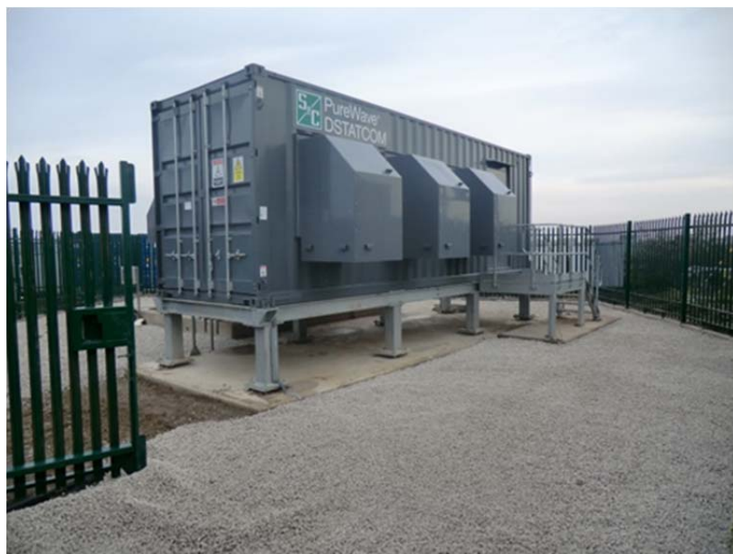
Figure 21 - DStatcom at Trusthorpe primary substation
