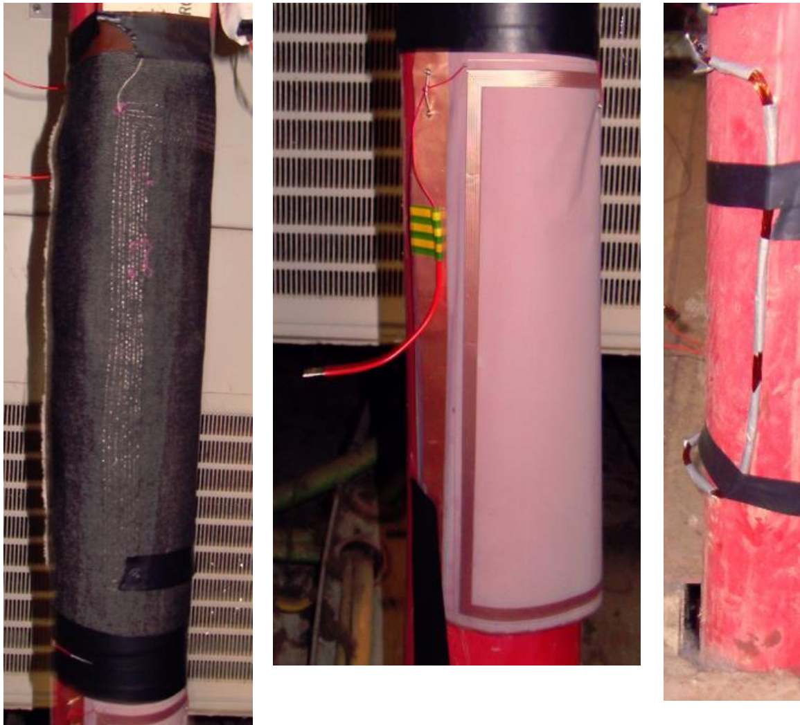
Figure 66: sewn , pcb and coil on substation cable
