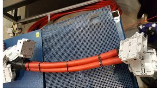
Figure 5: 11kV 3-core Trefoil XLPE cable
