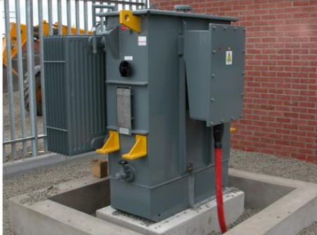
Figure 2 Photograph showing 11kV:230/400V oil cooled transformer
