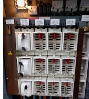
Figure 3 Photograph showing maximum demand indicators (top right), disconnector (right), rows of fuse holders with only 1 circuit (left hand circuit) fused.
