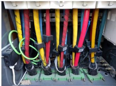
Figure 4 Photograph showing outgoing cables.
