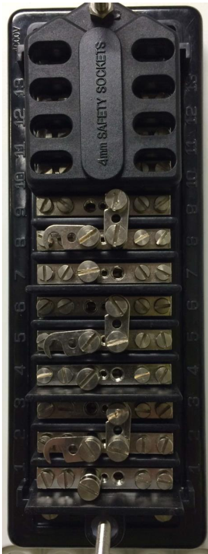
“METER” LINKS OPEN (Meter Disconnected From CTs)
