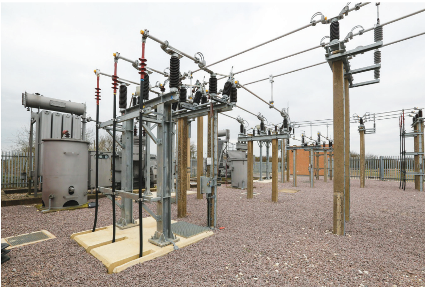
Figure 12 – Chapel St Leonards Installation – cable connections shown left of centre.
