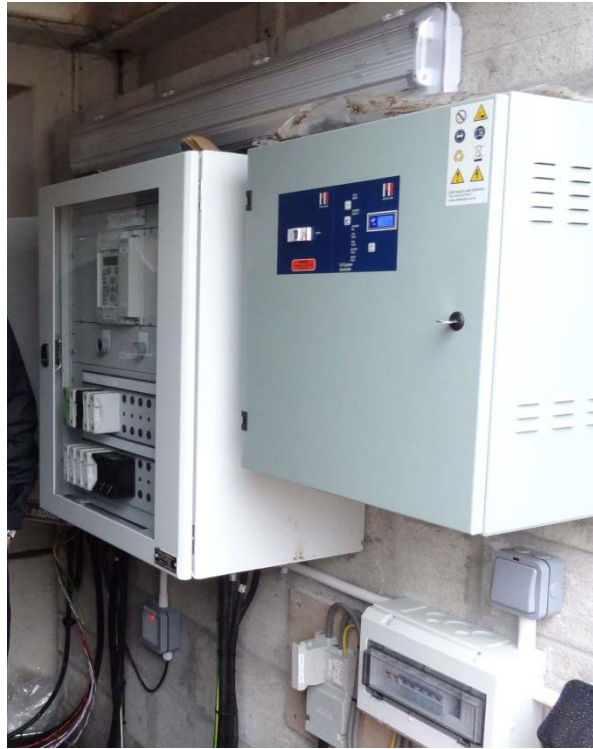
Figure 4: Voltage protection relay, battery and battery charger in situ
