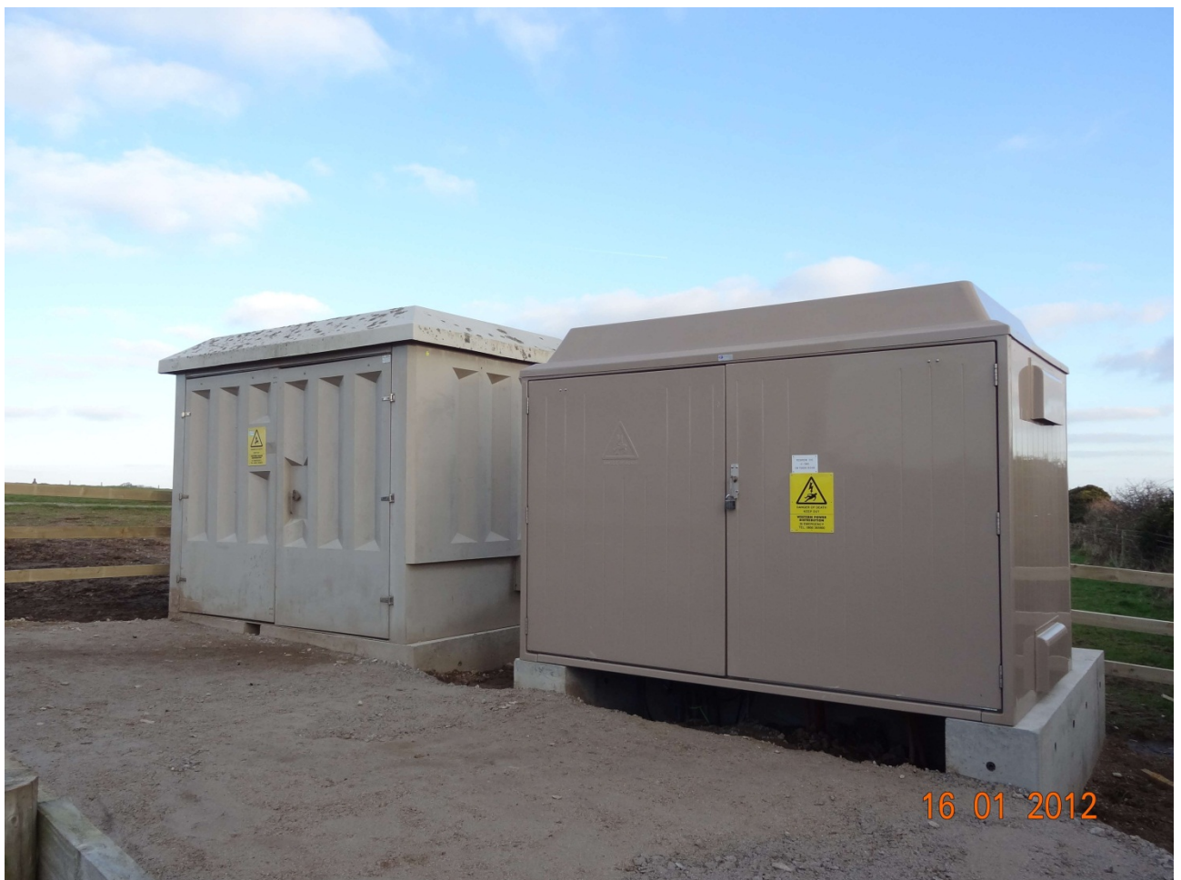
Figure 8: D-SVC (left) and associated transformer (right) installed on site
