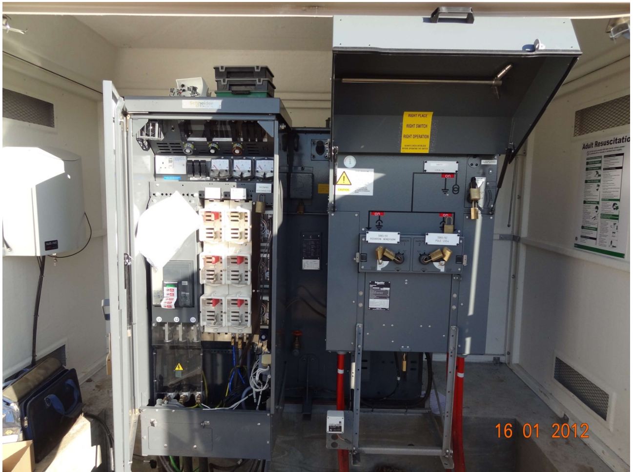
Figure 5: The D-SVC's dedicated transformer
